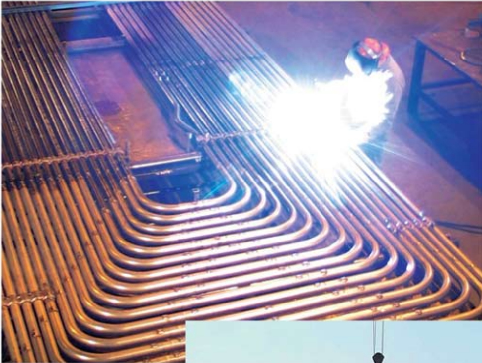
◀ Superheater for recovery boiler
